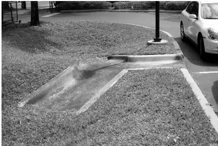
Figure 19.10 Alternative inlet bypass structure with low and high flow routes, Orlando, Florida, (courtesy Robert Bray Associates)
