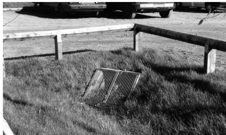
Figure 19.13 Photograph of screened orifice outfall with T-piece structure (courtesy Robert Bray Associates)
