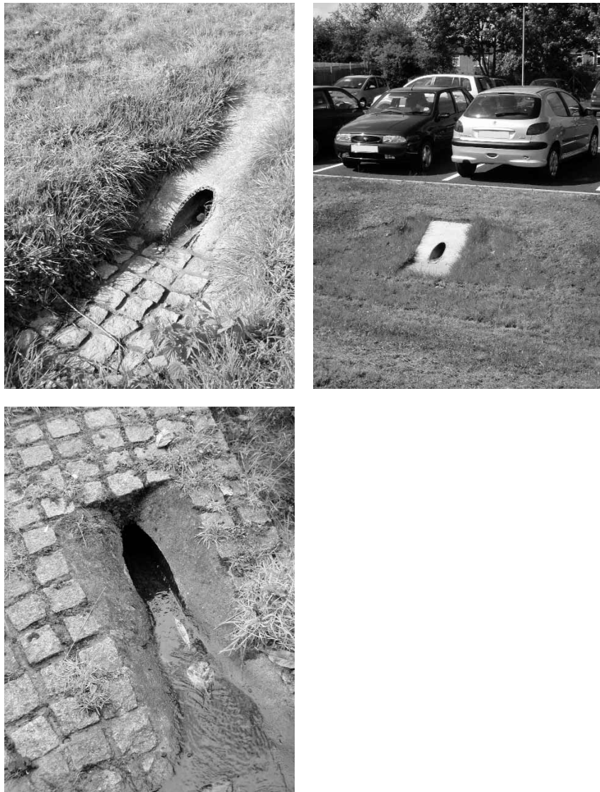
Figure 19.4 Photographs of low-flow inlet pipes to SuDS systems (courtesy Robert Bray Associates)
